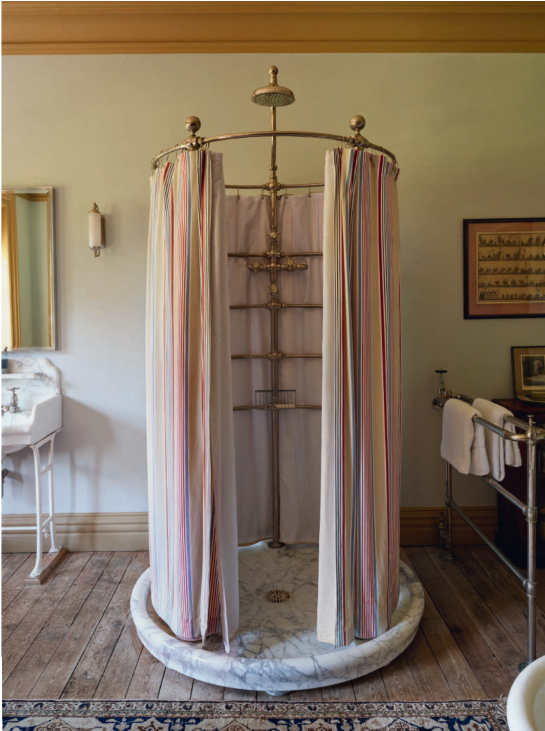
Above: the rib-cage shower, like all of the antique bathroom fittings in the house, is from Mongers, a salvage yard in Hingham, Norfolk. By necessity, the house's sanitaryware is Victorian, given that flushing loos were not patented until 1775. Opposite: the exquisite William & Mary-style tester bed, incorporating fragments of 17th-century damask, was bought from the Cowdray Park estate sale at Christie's in 2011. Visible beyond is an image of a penitent Mary Magdalene garlanded by flowers, attributed to the circle of the Neapolitan Luca Giordano
